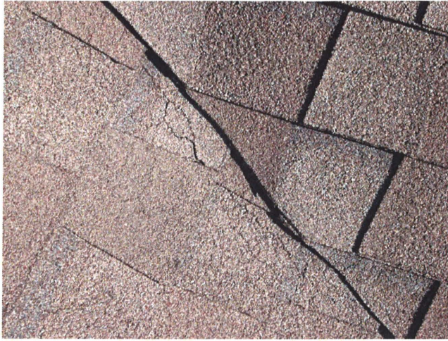
7. CRACKED SHINGLES IN VALLEY
