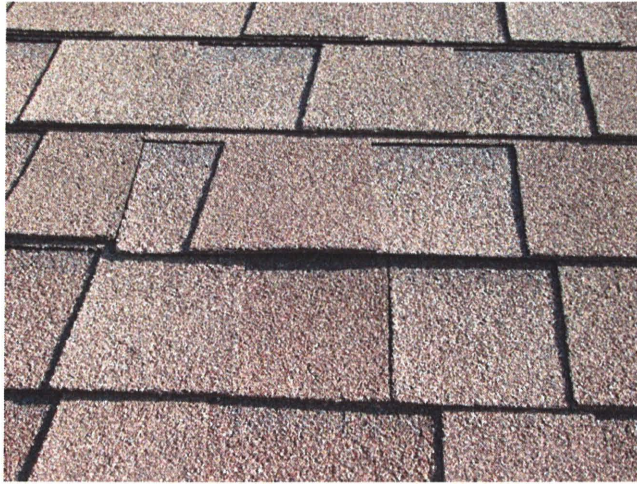
10. BACKED OUT FASTENER
