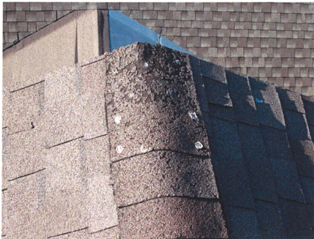
8. DETERIORATED RIDGE CAPS (TYPICAL)
